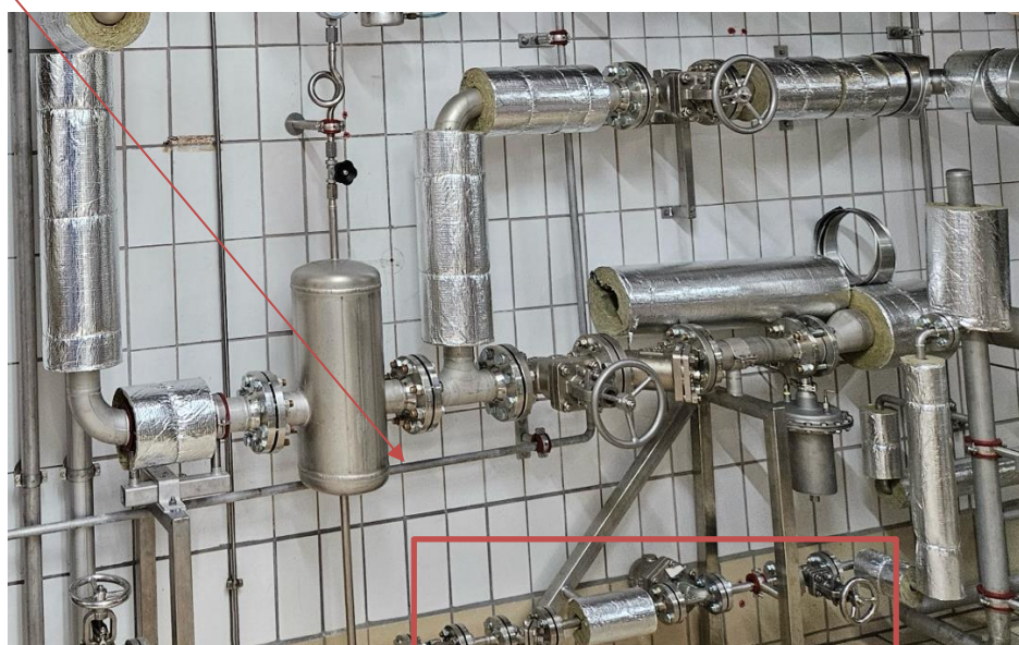
Figure 30 : Installation Despraz FX201
